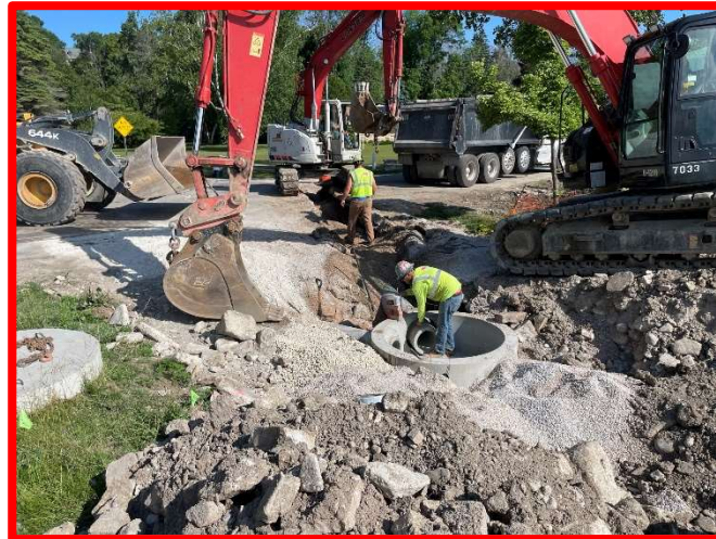
Figure 1: MJ construction installing a storm manhole near the intersection of Beach Dr and Beach Ct
