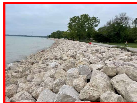
Figure 3: A view of the completed revetment on the south end of the project.
