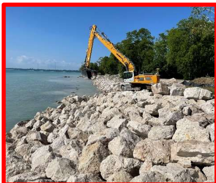
Figure 2. Michel's installing armor stone on the north end of the northern portion of the project.
