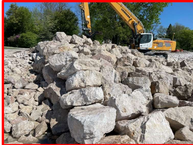
Figure 1: Excavator equipped with GPS technology used to place the revetment stone at the exact right location and elevation. Pictured above creating a trench for storm sewer to be installed.
