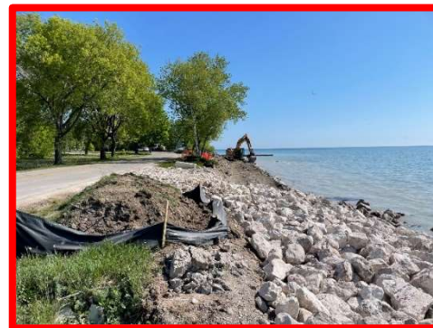
Figure 3: Second excavator equipped with GPS technology clearing debris and preparing the base layer for installation of the armor stone.
